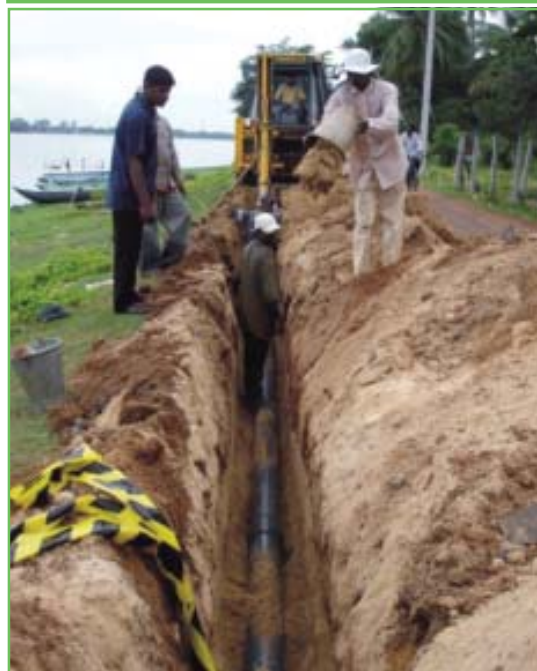
Figure 35: Oxfam laying pipes for water connections to hand over to the Batticloa Water Board
